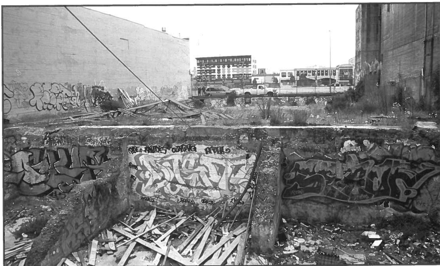
This site of the old Embassy Theater on Market Street between Seventh and Eighth Streets has been vacant since its demolition following the Loma Prieta earthquake. The new Federal Building will be built on the site of the former Greyhound terminal, in the background, and will form a wall between this site and Mission Street.
