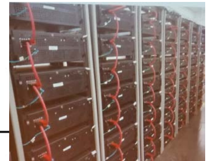
Smart Microgrid + Second life Li-Ion Energy Storage
